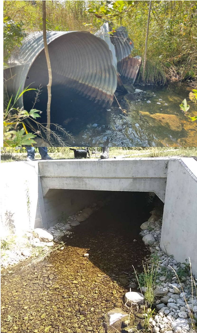
Figure 5. Before and after (2023) pictures of Boyer Road-Tannery Creek crossing. This crossing is between TYC1B and TYC2A.
