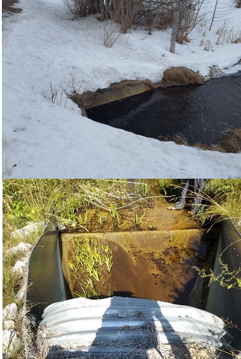
Figure 7. Before and after (2023) pictures of Mitchell Road-Tannery Creek crossing. This is the next road upstream of TYC2A.
