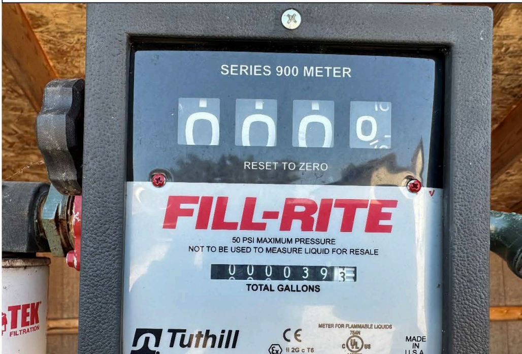
Photo 2: A view of the meter for the green AST.
