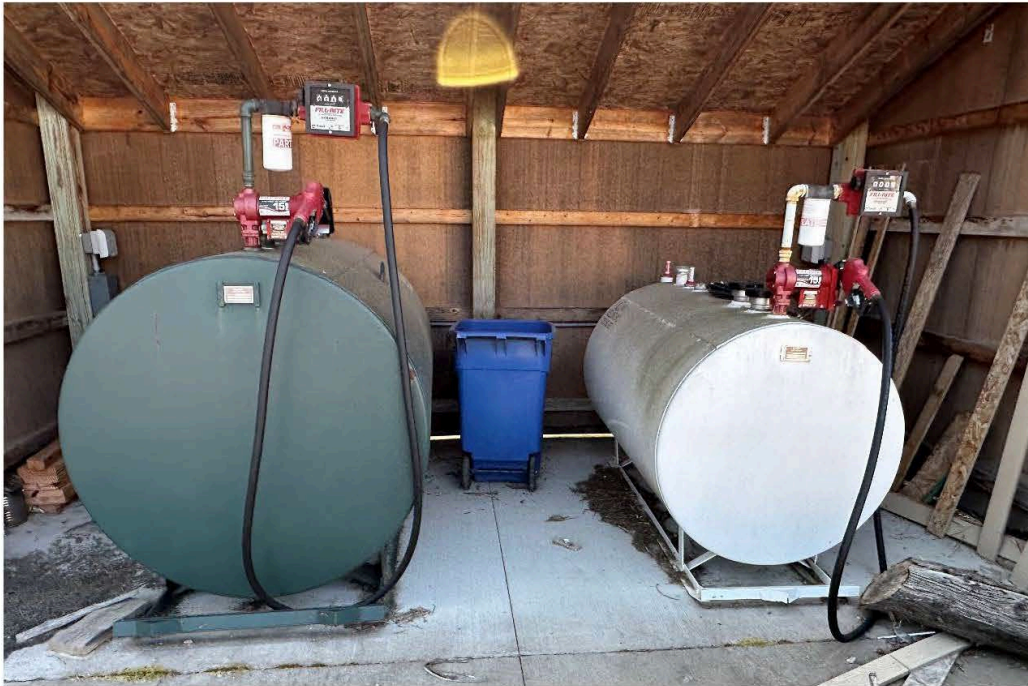
Photo 1: A view of the two ASTs that will need to be emptied (if any product remains inside) and flushed/cleaned so that they can be sold or reused for other product.
