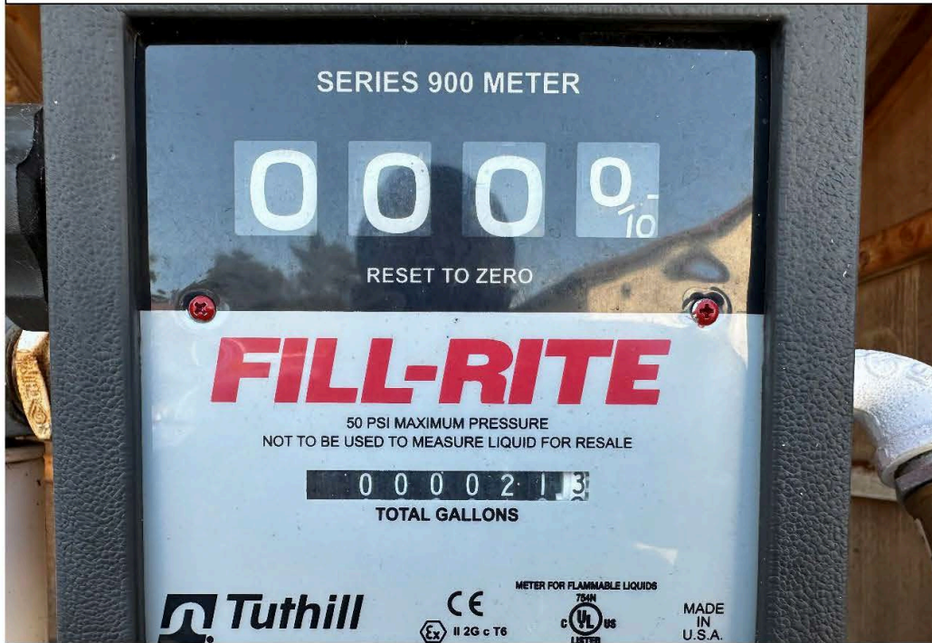
Photo 4: A view of the meter for the smaller white AST.
